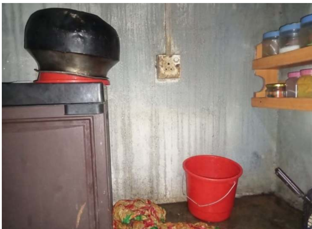
Image 20: Owner: deteriorating conditions in the home due to water leaks
