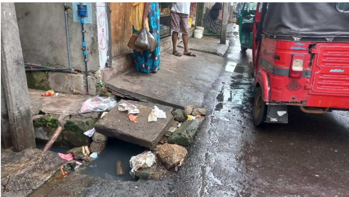
Image 29: Blocked and overflowing drains, captured by agent, member of Samurdhi welfare society
