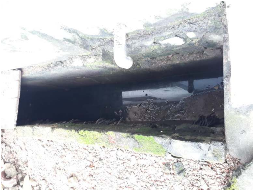
Image 27: Encroached: Open drains prone to mosquito breeding
