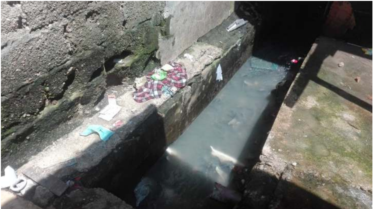
Image 25: Tax deed: Dirty water in drains
