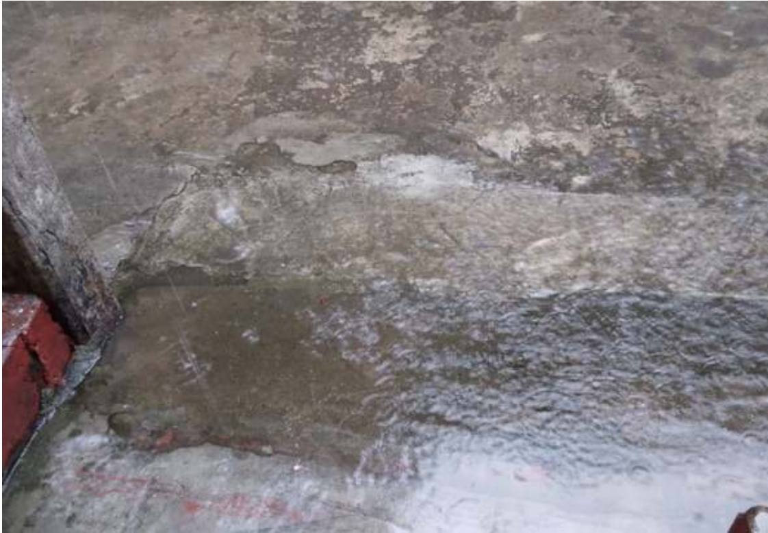
Image 26: Renter: Floods due to raining
