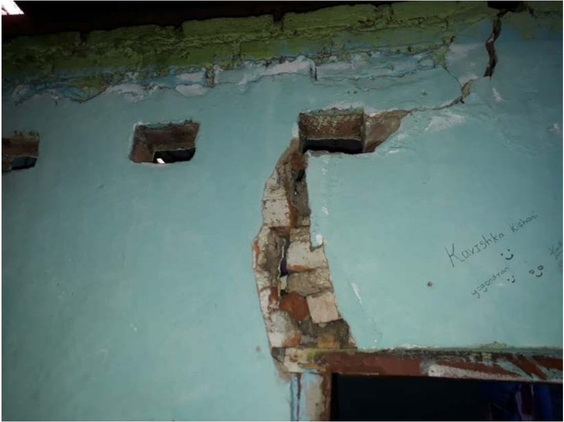
Image 21: Renter: cracks on wall in a rental home
