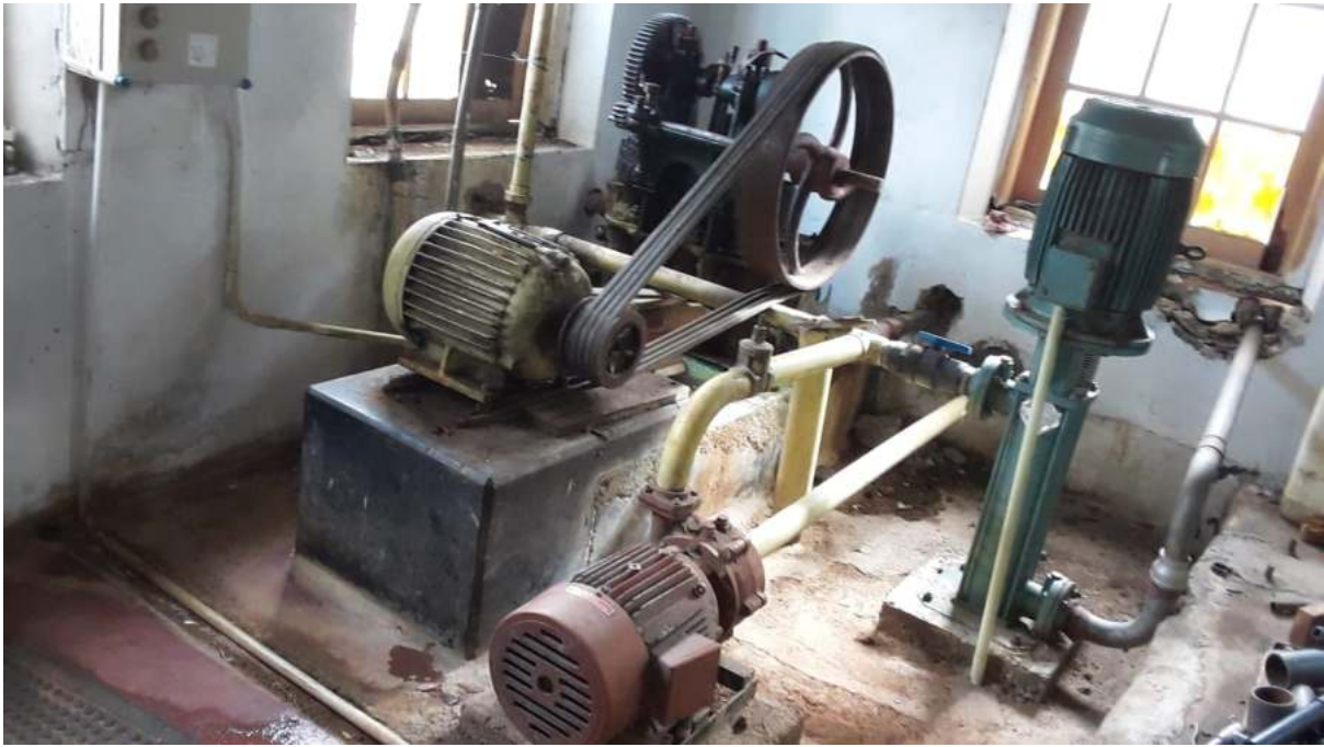
Image 5: Photo by agent, water distributor, of an outdated motor system to pump water in Sarnia
