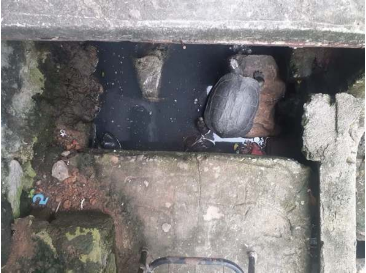
Image 24: Owner: Unsanitary drainage systems that overflow during floods
